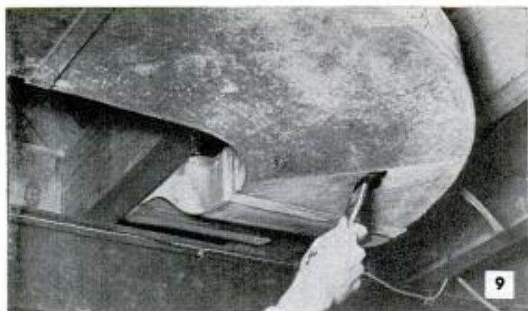
In time, rust will work through the protective galvanizing on ducts of the heating system. Aluminum paint is added protection
